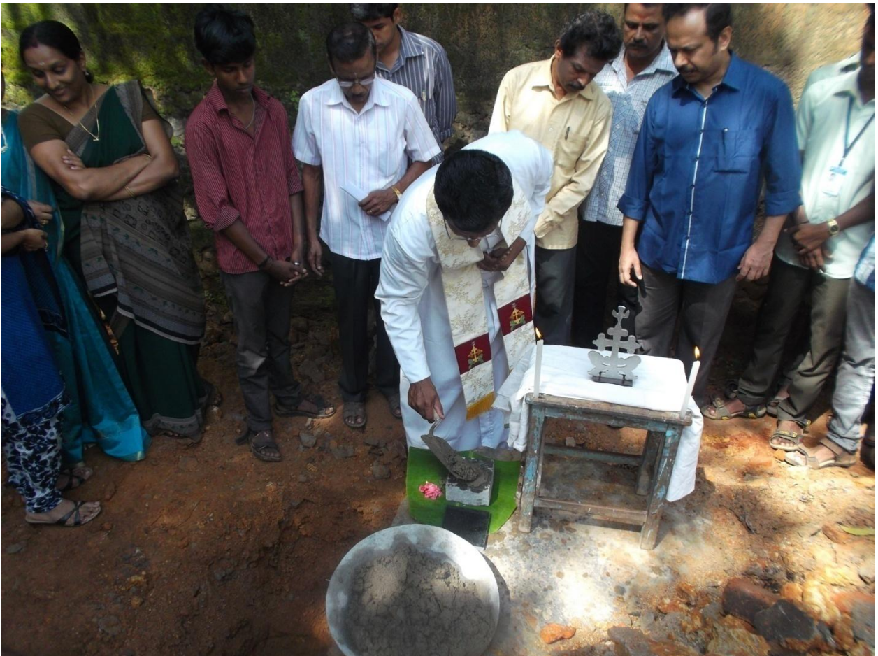
The laying of foundation stone for NSS Bhavan at Athirampuzha on 31 st October 2014
